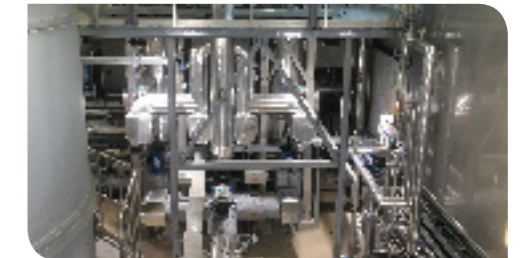
Exleys ™ , Settled in Yeosu STP
